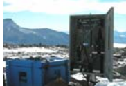
Site TM1 instrumentation. The array is buried 2m to the right. The blue box houses batteries.
