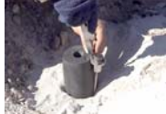
Installation of thermal array (thin metal tube). Surface debris was then restored to original state.
